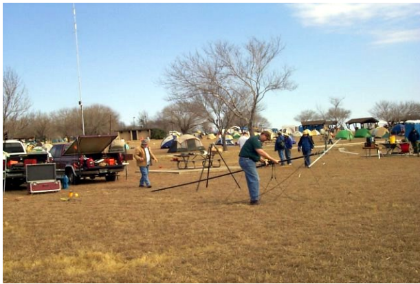
D.C. and Brad setting up the VHF antenna
